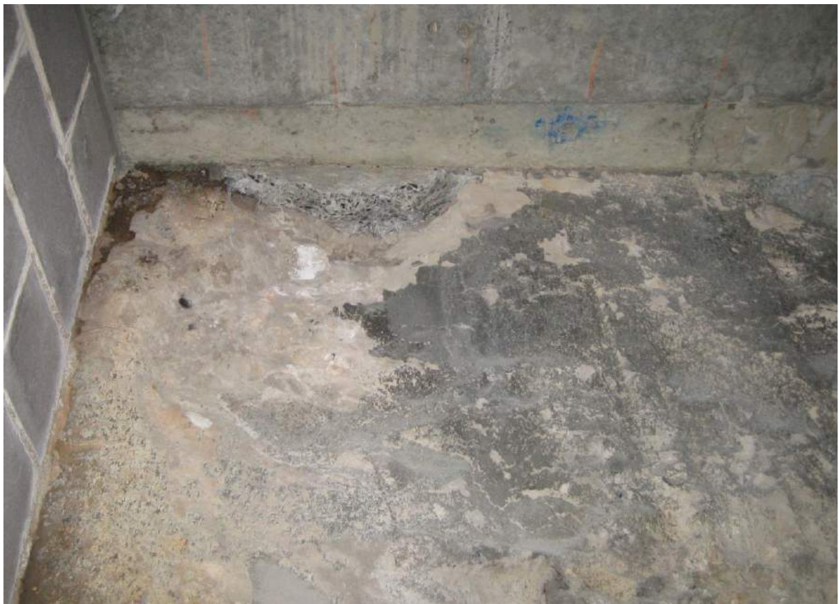
Photo No. 68: Spalling of wall in fire stair walkway on western side of garage on Level B1.
