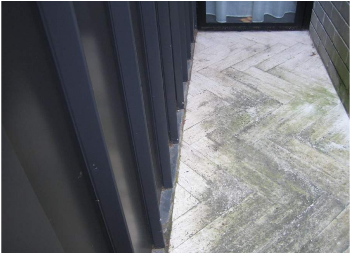
Photo No. 49: Tiled balcony return adjacent water leak in bedroom 2 in Unit 407.
