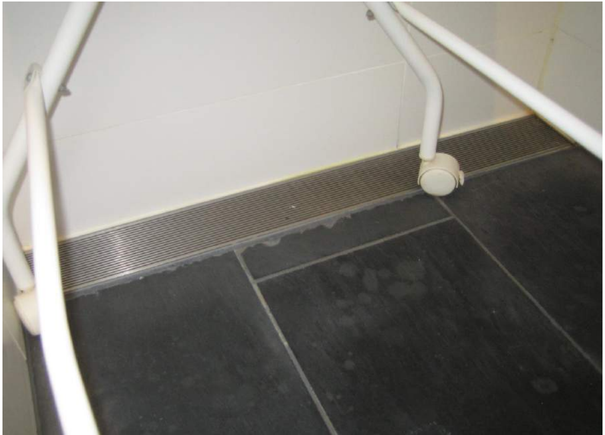
Photo No. 31: Water ponds on shower cubicle floor in bathroom and does not drain in Unit 311.
