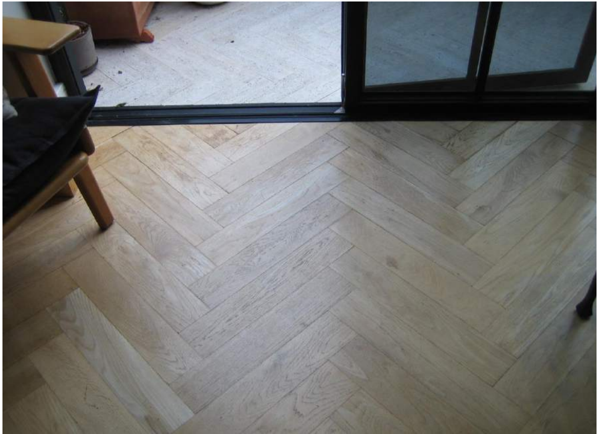
Photo No. 41: Water penetration and damage to the living room timber floor areas in Unit 406.
