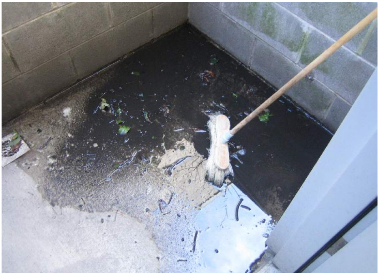
Photo No. 72: Water ponding on landing to A/C units outside Waste Room in Building B.
