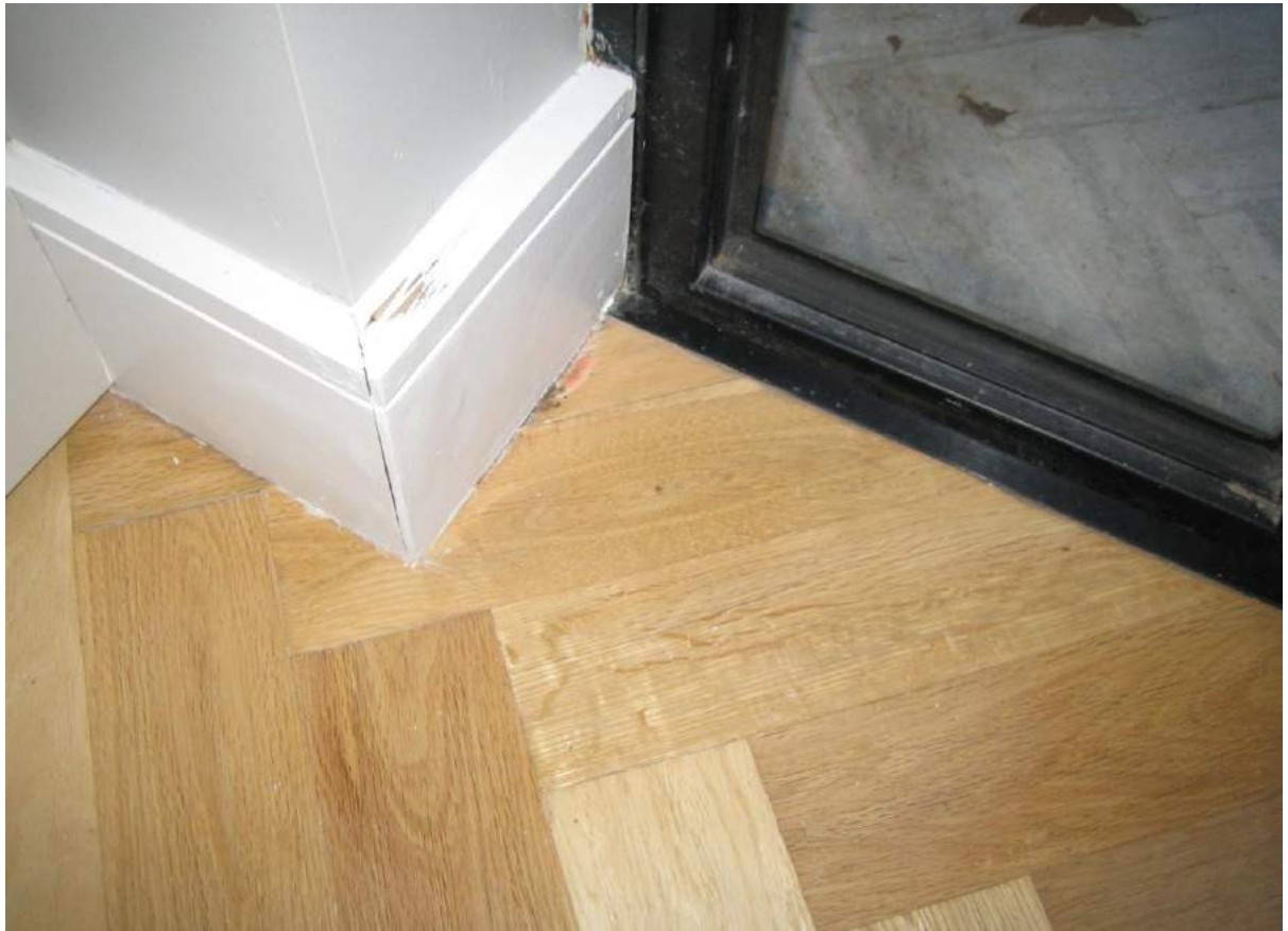
Photo No. 3: Water penetration and damage in northern corner of bedroom 2 in Unit G01.
