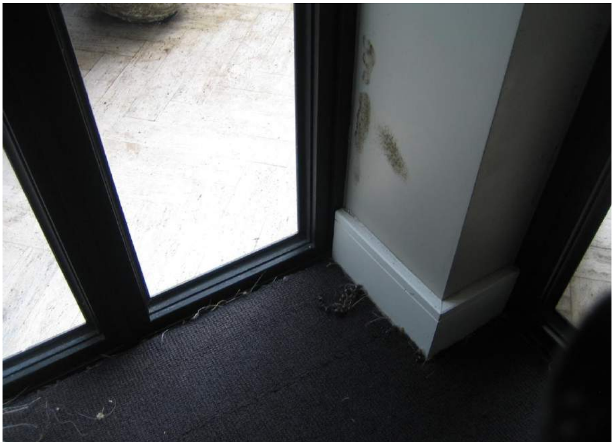
Photo No. 4: Water penetration, damage and mould in N/E corner of bedroom 1 in Unit G05.
