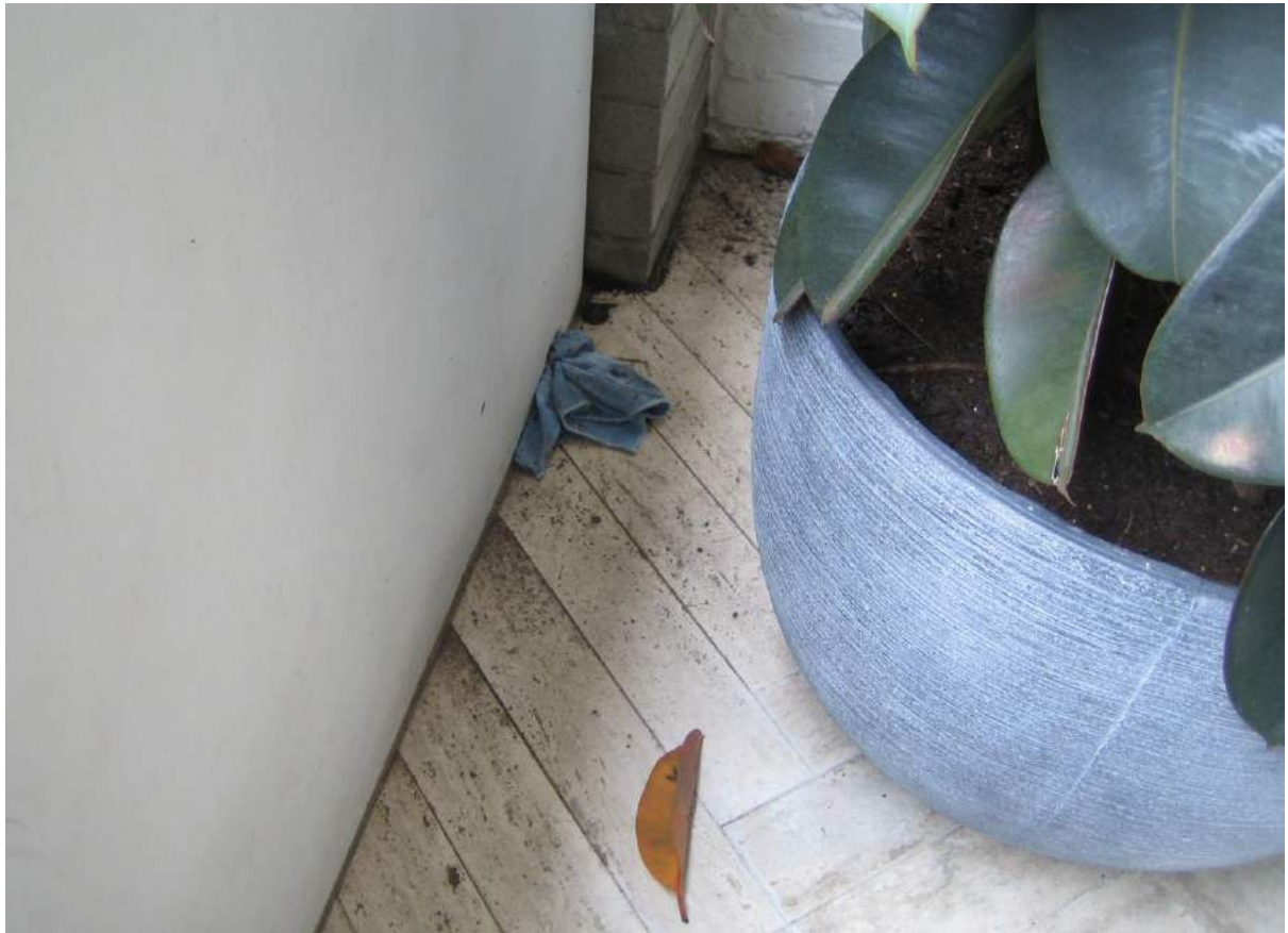
Photo No. 33: Water on balcony does not drain to floor waste but drains to spitter in Unit 311.
