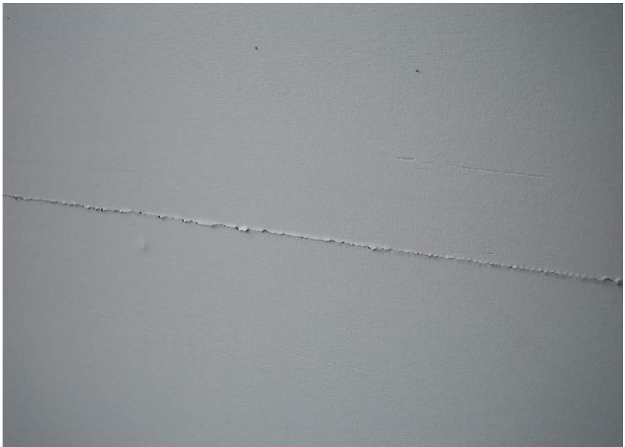
Photo No. 36: Cracked horizontal taped joint on the eastern balcony wall in Unit 404.
