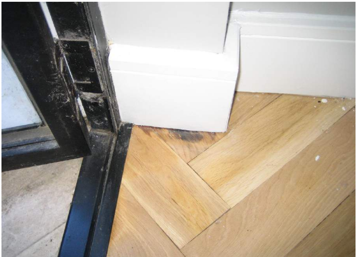
Photo No. 2: Water penetration and damage in N/W corner of bedroom 1 in Unit G01.
