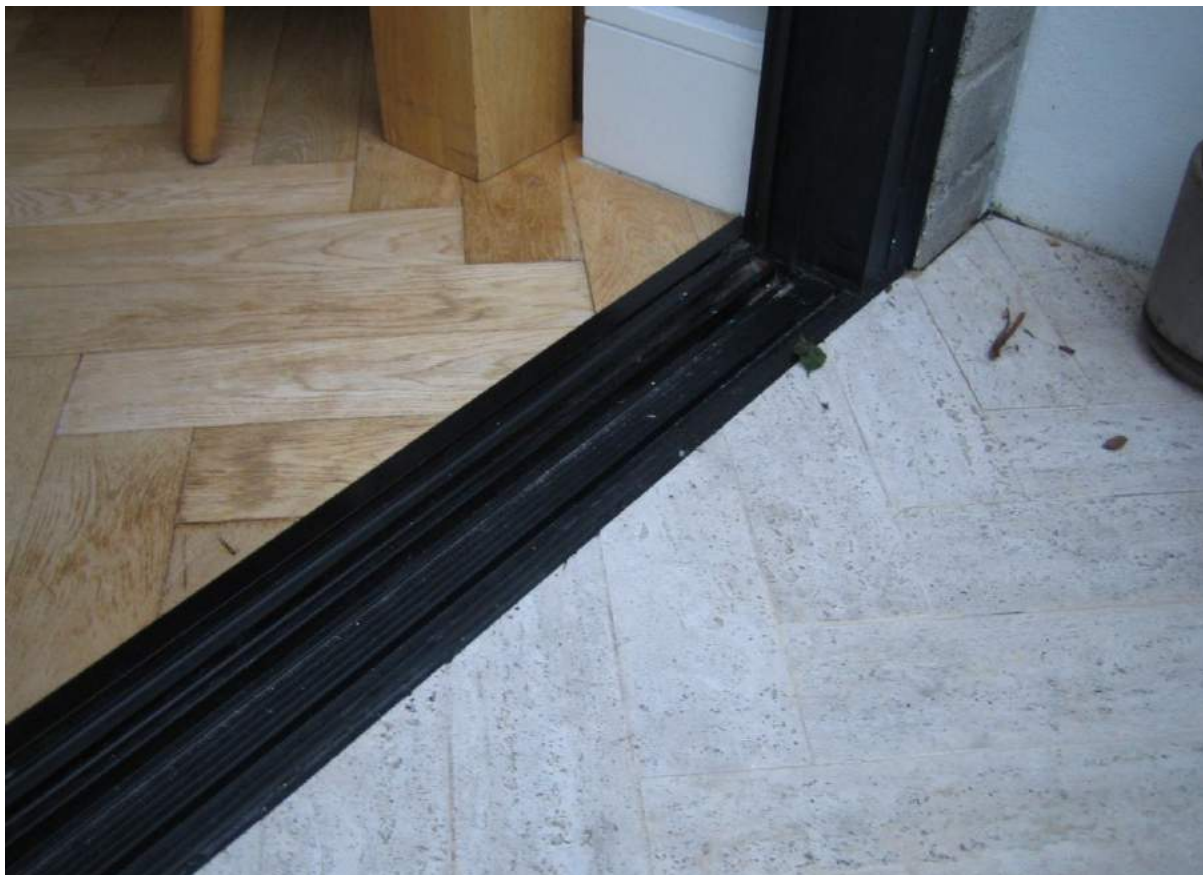
Photo No. 40: Water penetration and damage at living room balcony doors in Unit 406.
