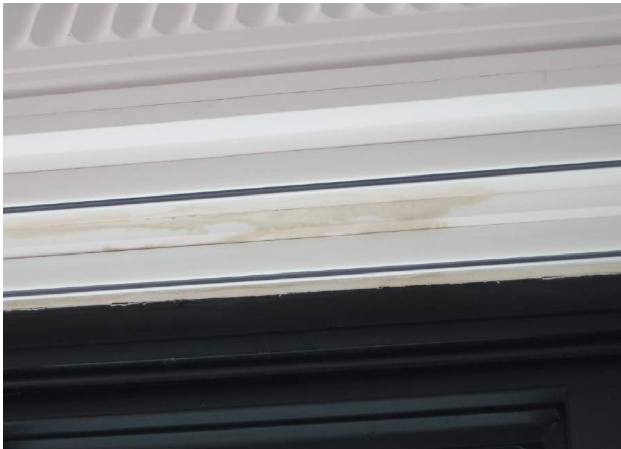
Photo No. 26: Water penetration in top centre of living room window assembly in Unit 306.
