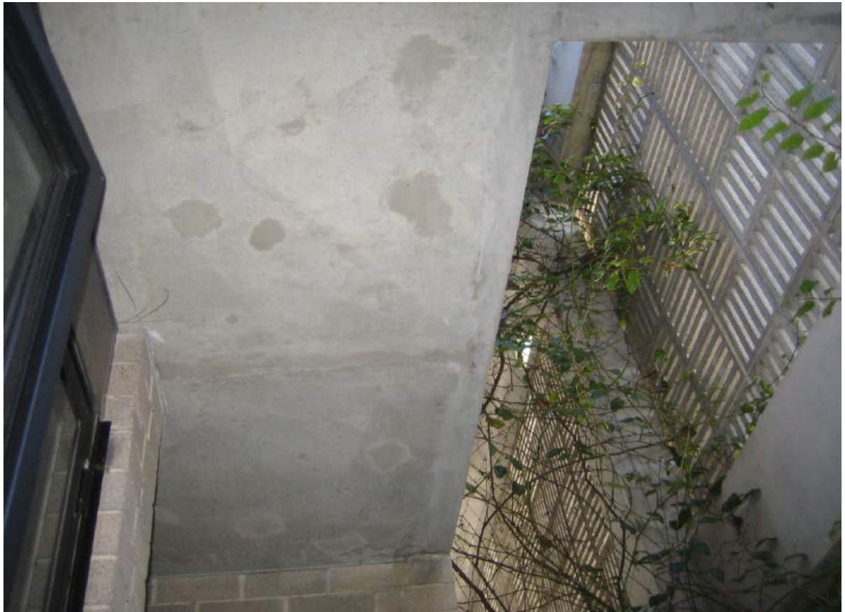
Photo No. 15: Soffit of balcony over bedroom 2 in Unit 207 has no drip-groove installed.
