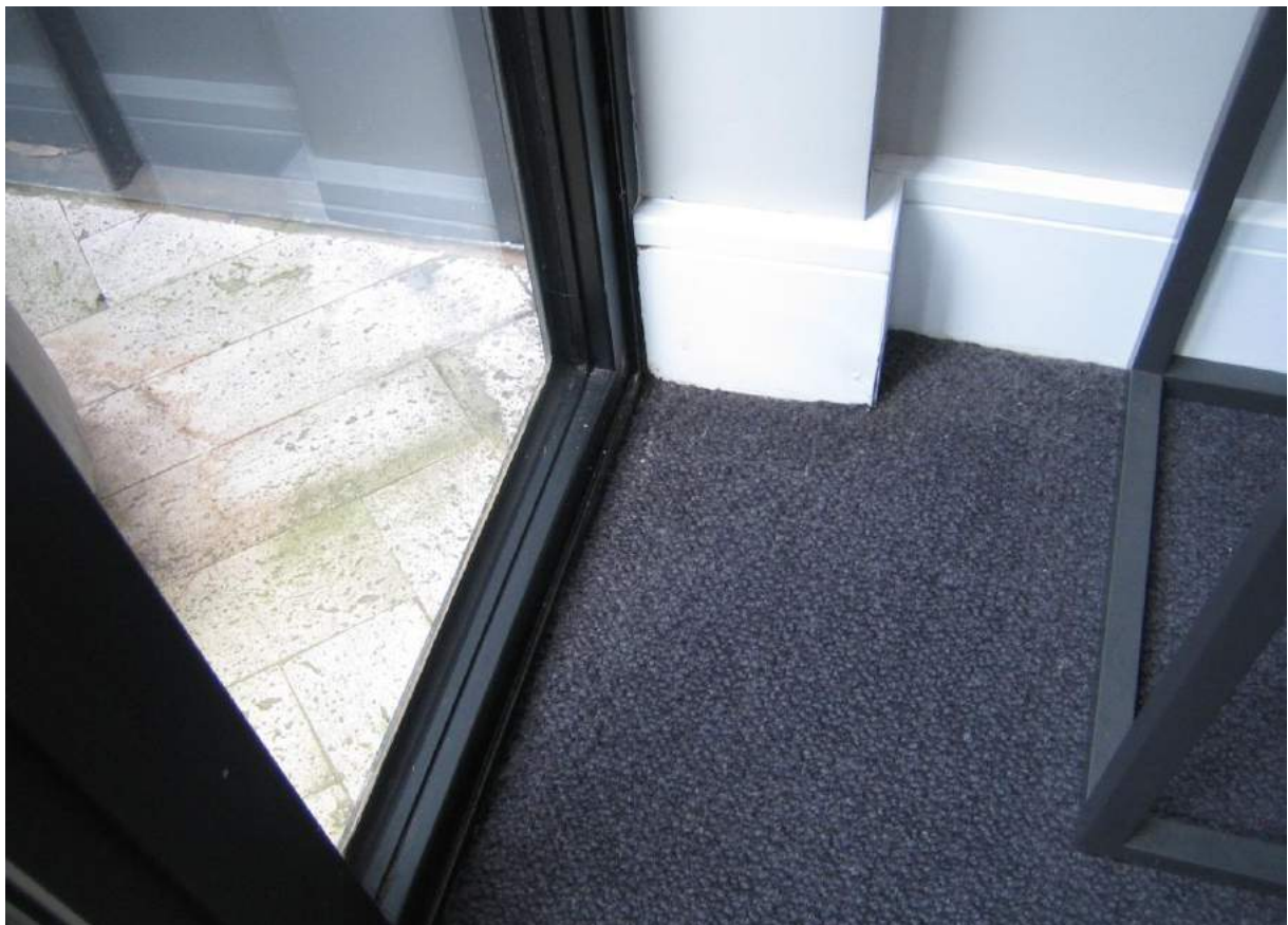
Photo No. 46: Water penetration and damage within bedroom 2 from balcony door in Unit 407.
