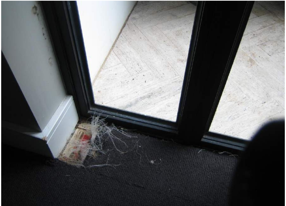
Photo No. 5: Water penetration, damage and mould in N/E corner of bedroom 1 in Unit G05.
