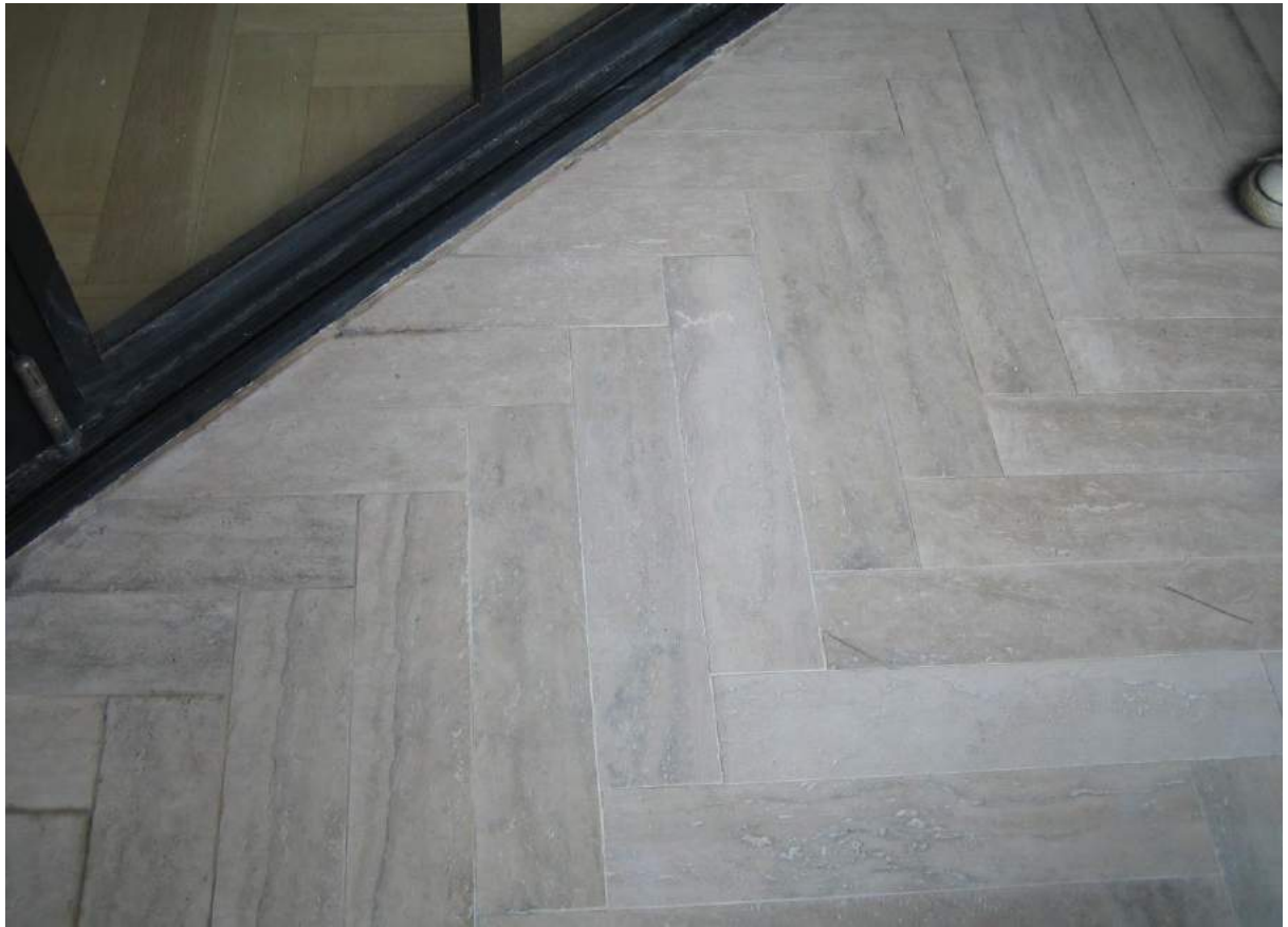
Photo No. 53: Repaired tiled area on the balcony off the living room in Unit 409.
