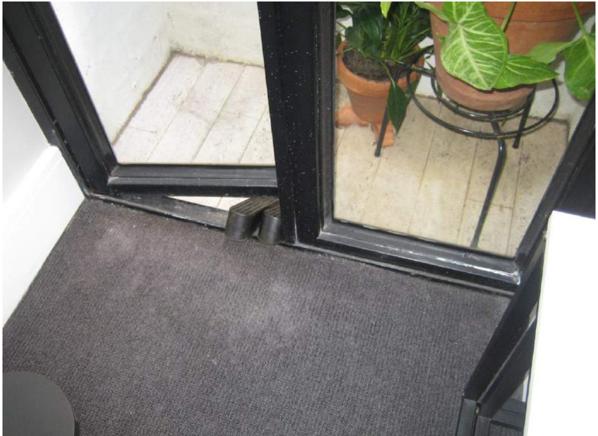
Photo No. 39: Water penetration and damage at the balcony door in bedroom 2 in Unit 405.
