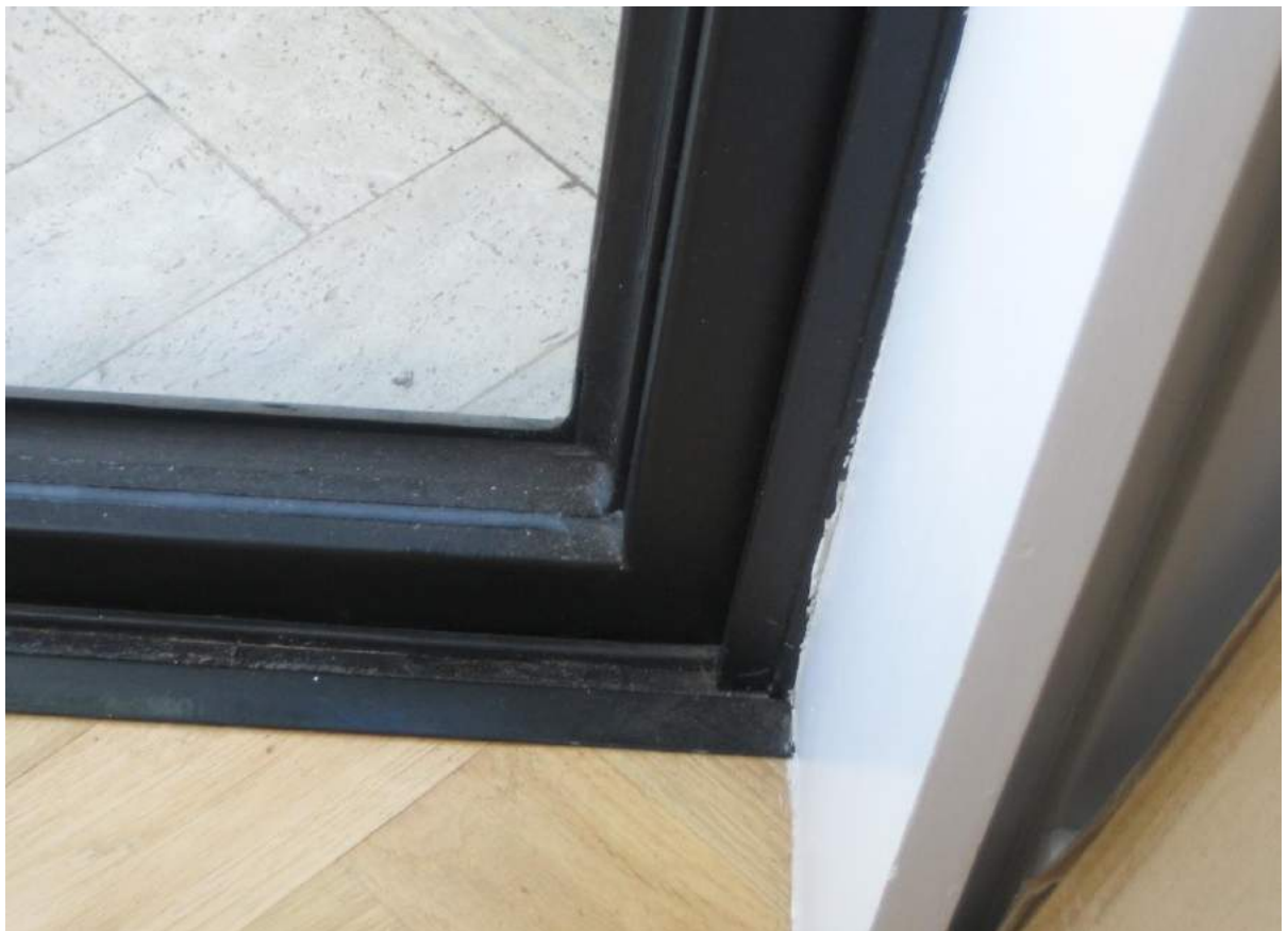
Photo No. 28: Water damage to parquetry flooring at eastern end of living room in Unit 306.
