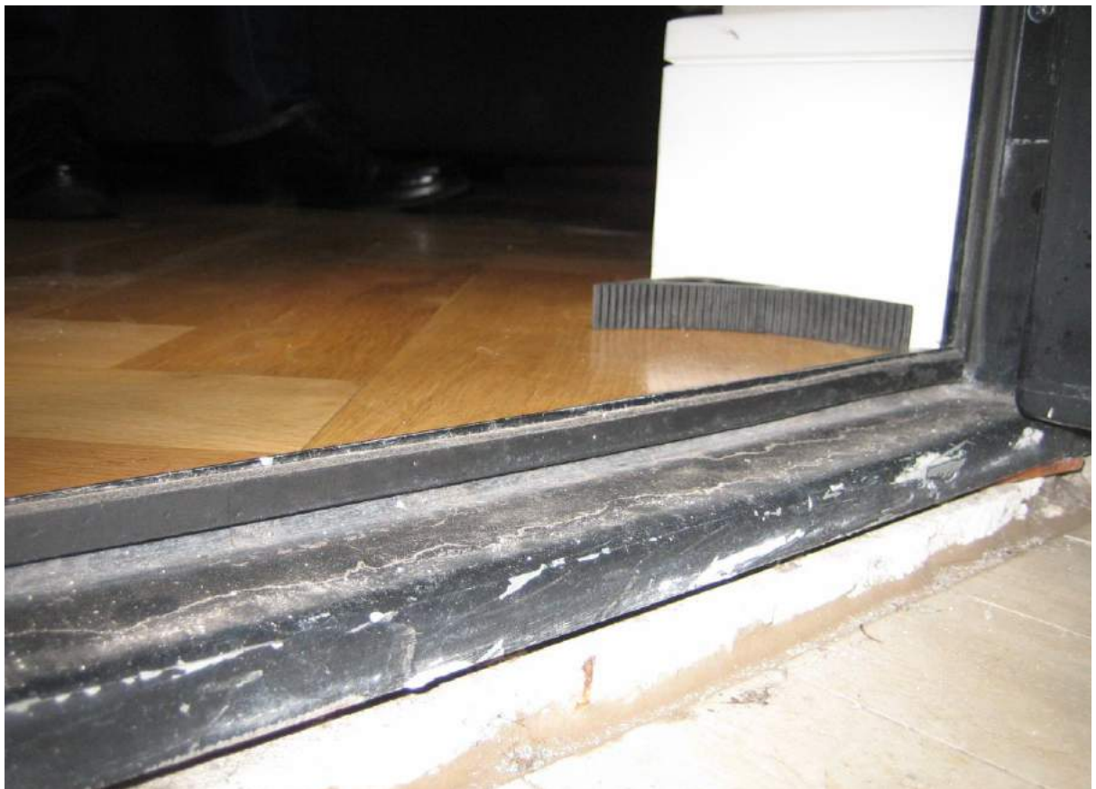
Photo No. 22 Incorrectly installed sub-sill to the French doors in bedroom 1 in Unit 303.
