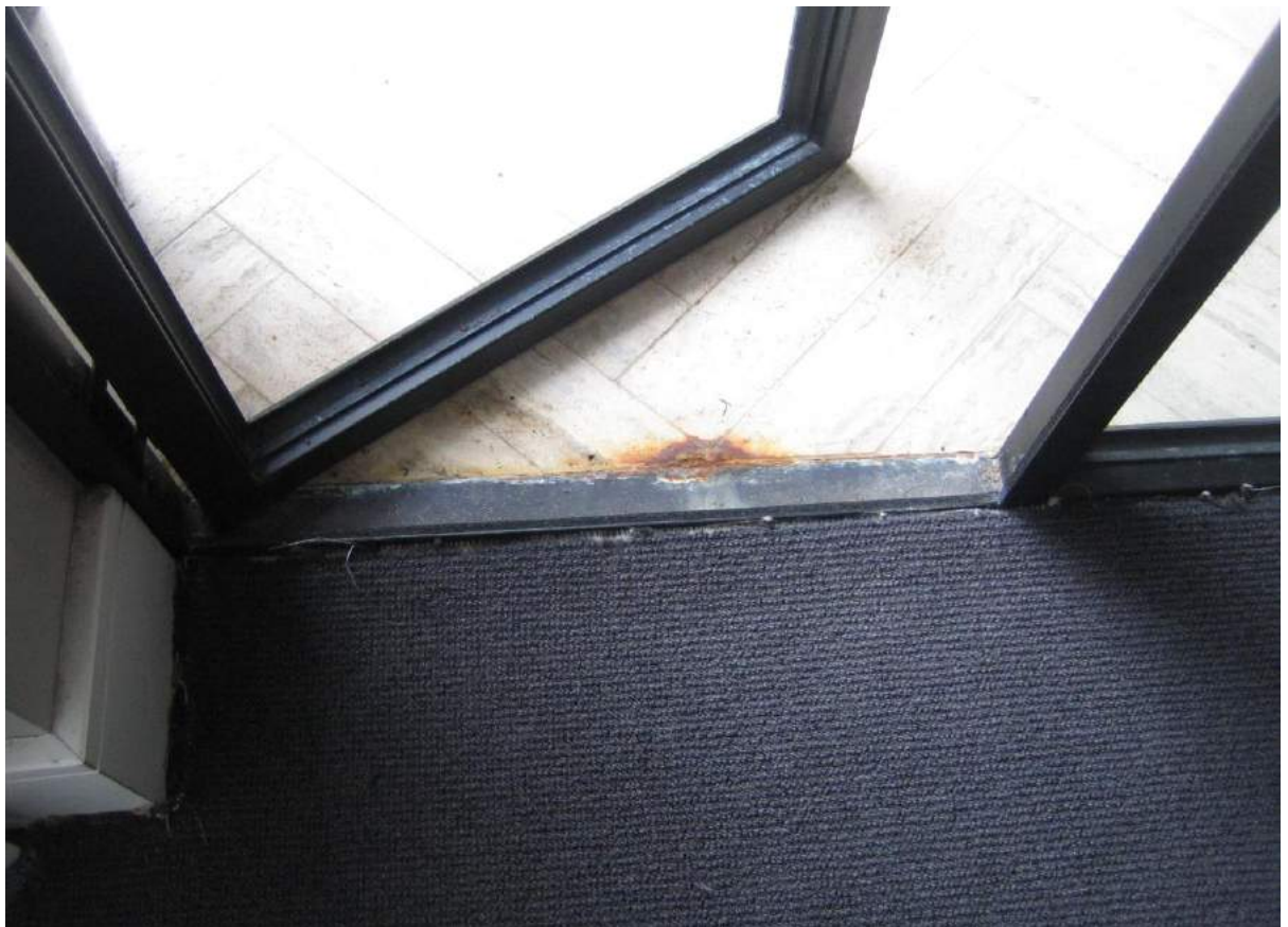
Photo No. 6: Corrosion in the base of glass door on northern side of bedroom 1 in Unit G05.
