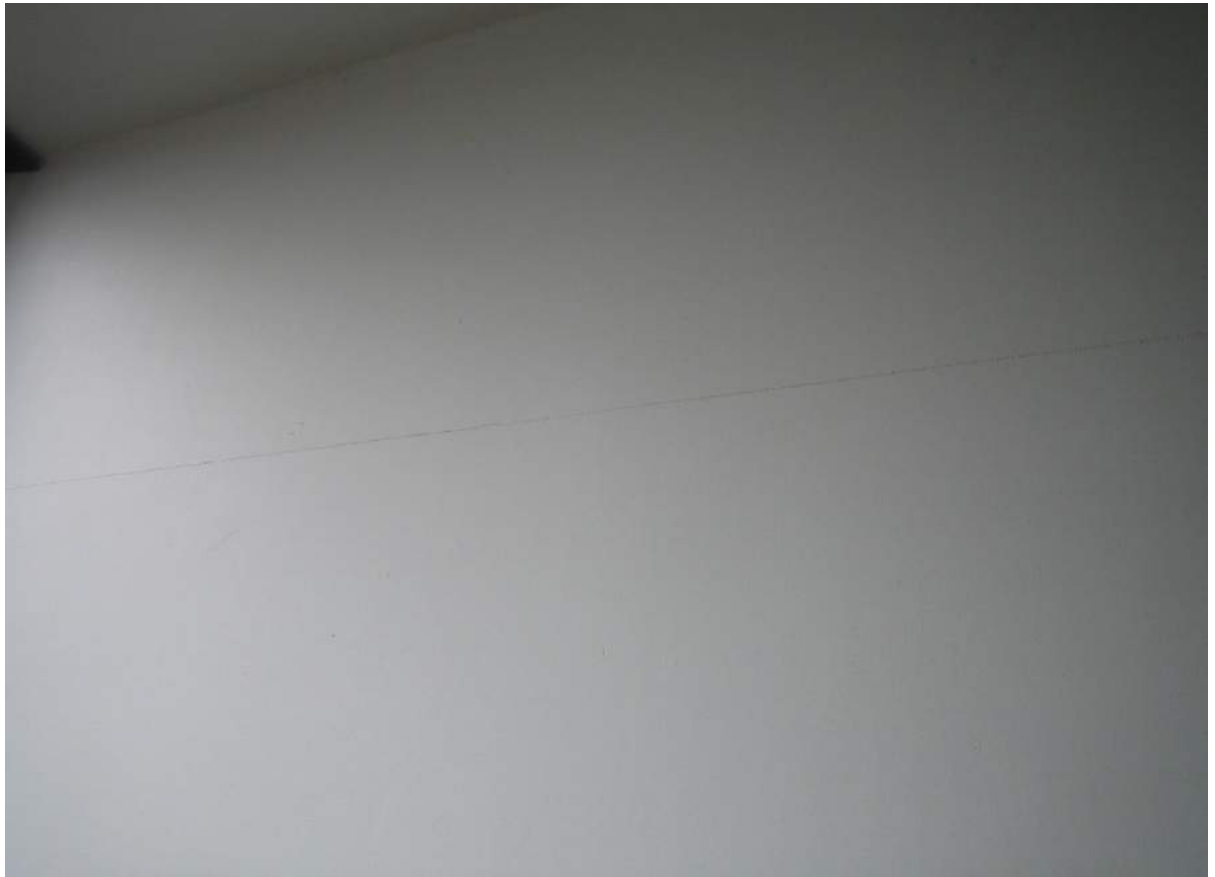
Photo No. 37: Cracked horizontal taped joint on the eastern balcony wall in Unit 404.
