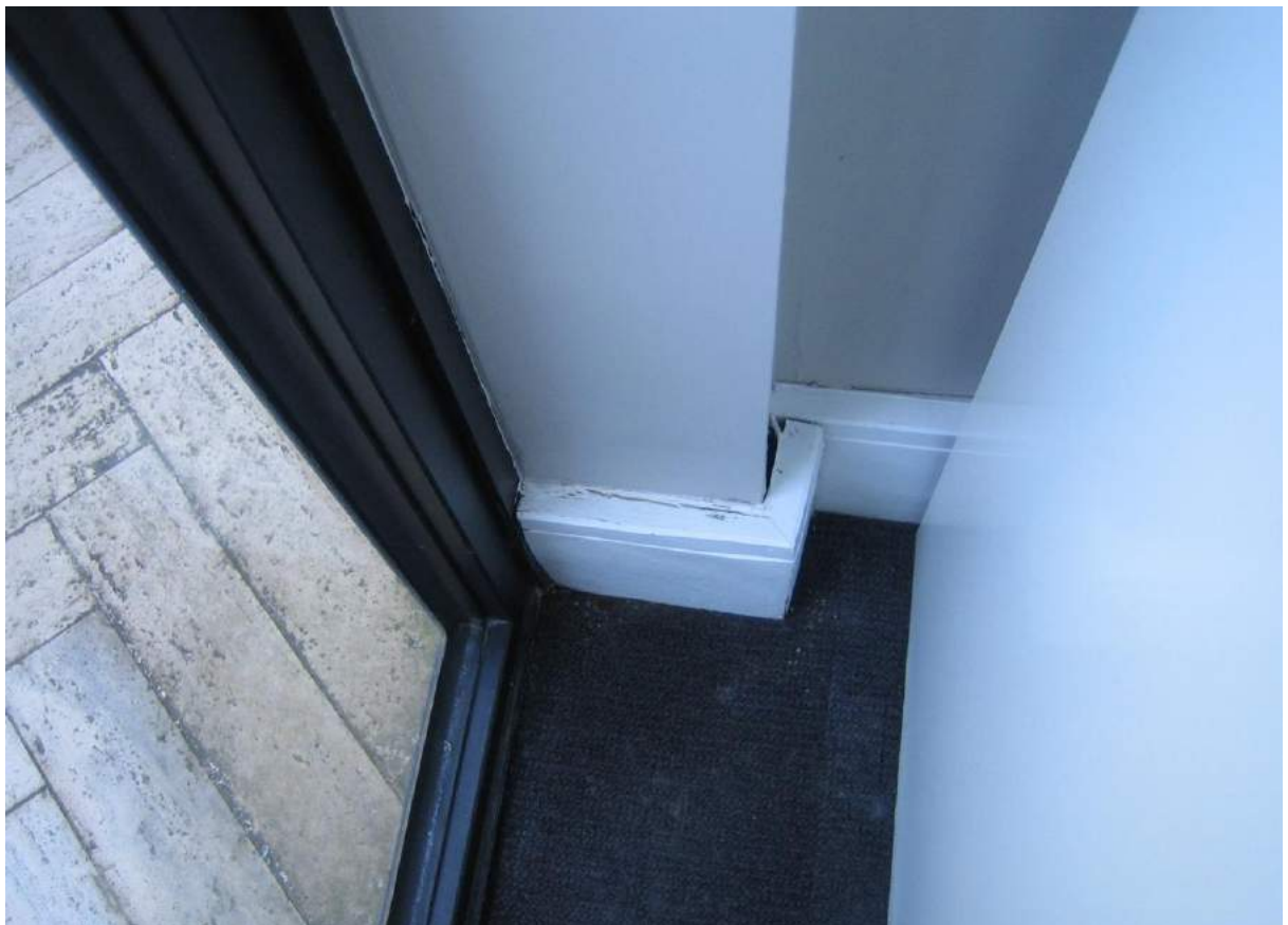
Photo No. 54: Water damage to skirting at western end of balcony door to Bed 3 to Unit 410.
