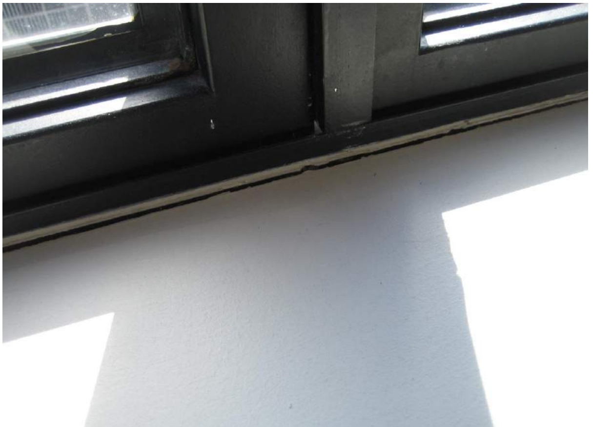
Photo No. 38: Water penetration in the window in the N/E corner of bedroom 1 in Unit 405.
