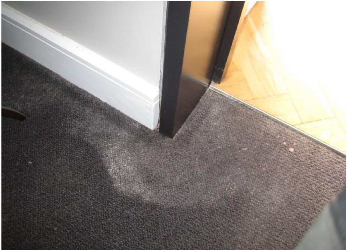
Photo No. 45: Water penetration and damage at the entry door to bedroom 1 in Unit 407.
