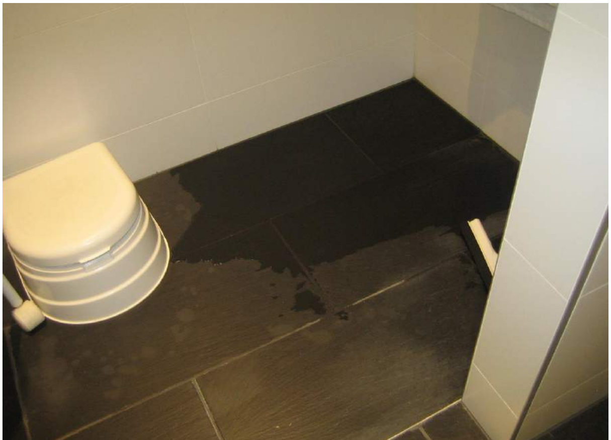
Photo No. 30: Water ponds on shower cubicle floor in bathroom and does not drain in Unit 311.
