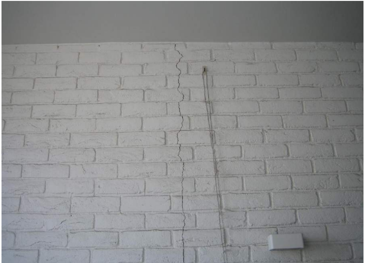
Photo No. 29: 1mm wide movement crack in the eastern balcony wall in 307.
