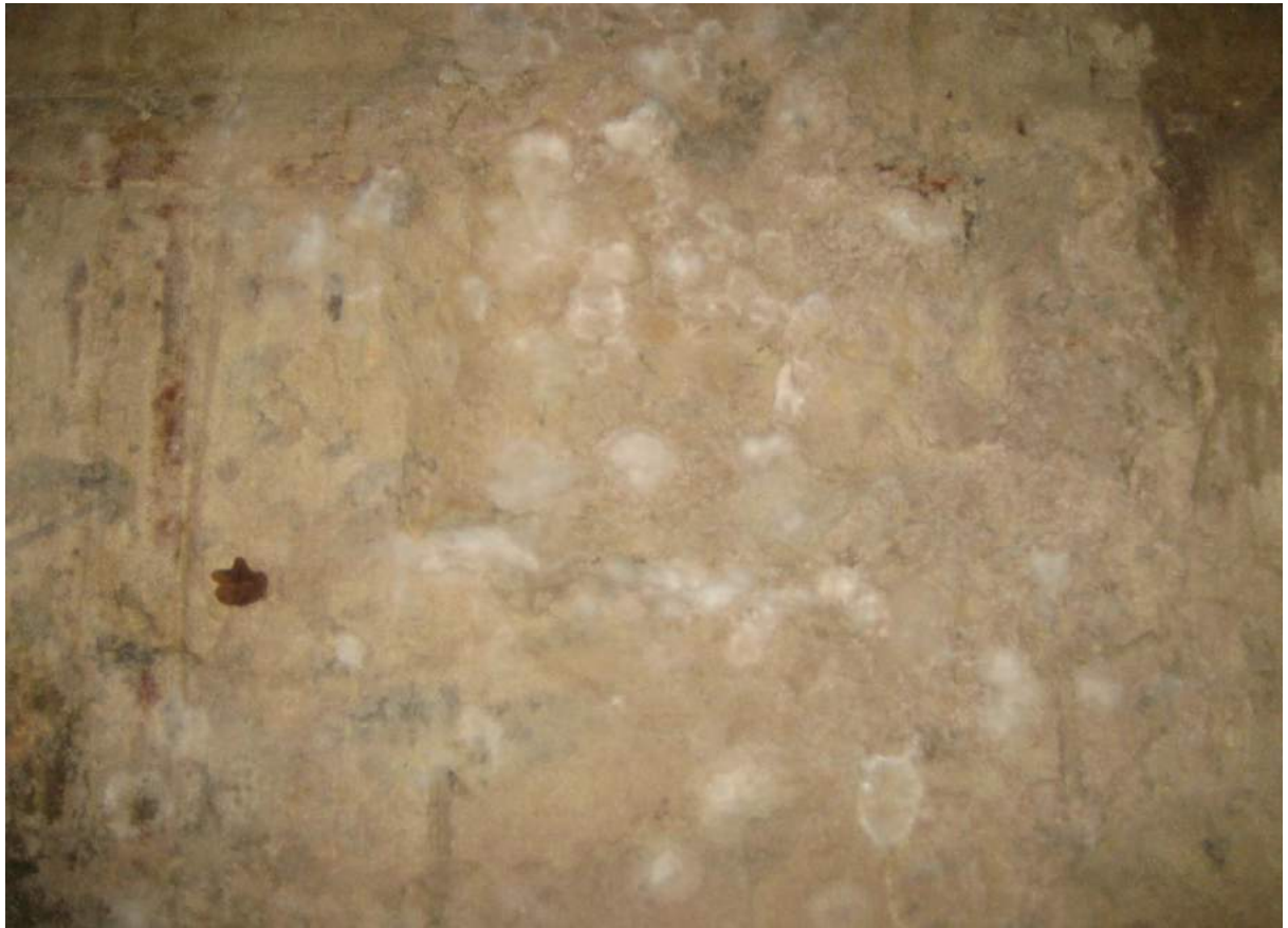
Photo No. 71: Heavy mould in fire stair walkway on the eastern side of garage on Level B1.
