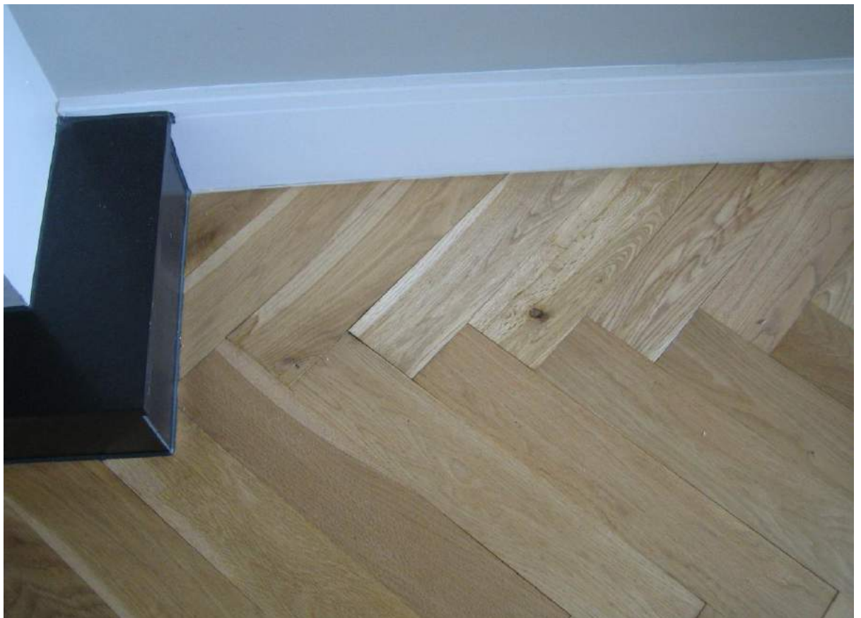
Photo No. 32: Parquetry flooring in living room is lifting due to possible ensuite leak in Unit 311.
