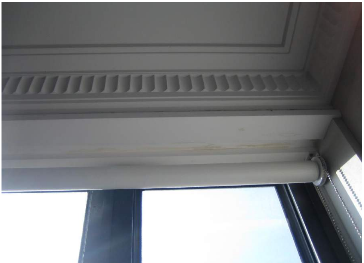
Photo No. 8: Water penetration in head of the eastern window in bedroom 1 to Unit 101.
