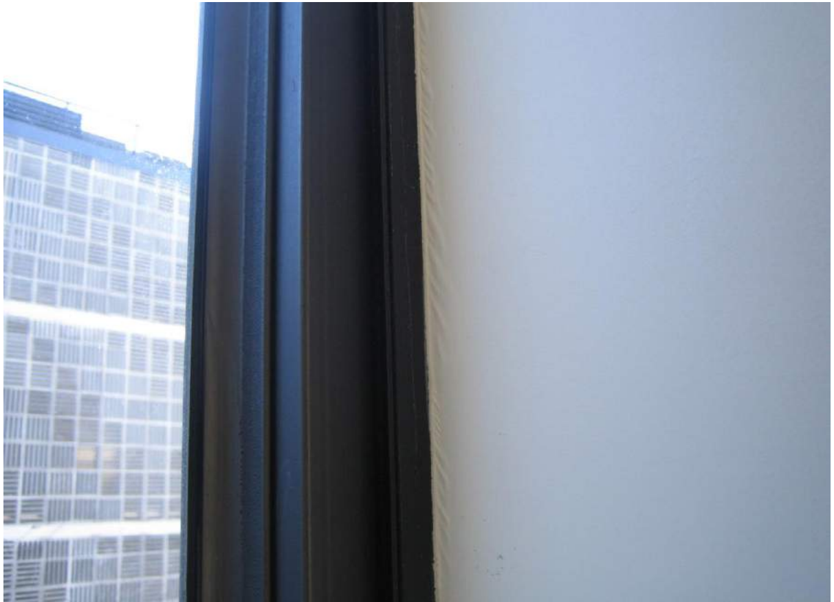
Photo No. 13: Water penetration in window in the N/E corner of bedroom 1 to Unit 205.
