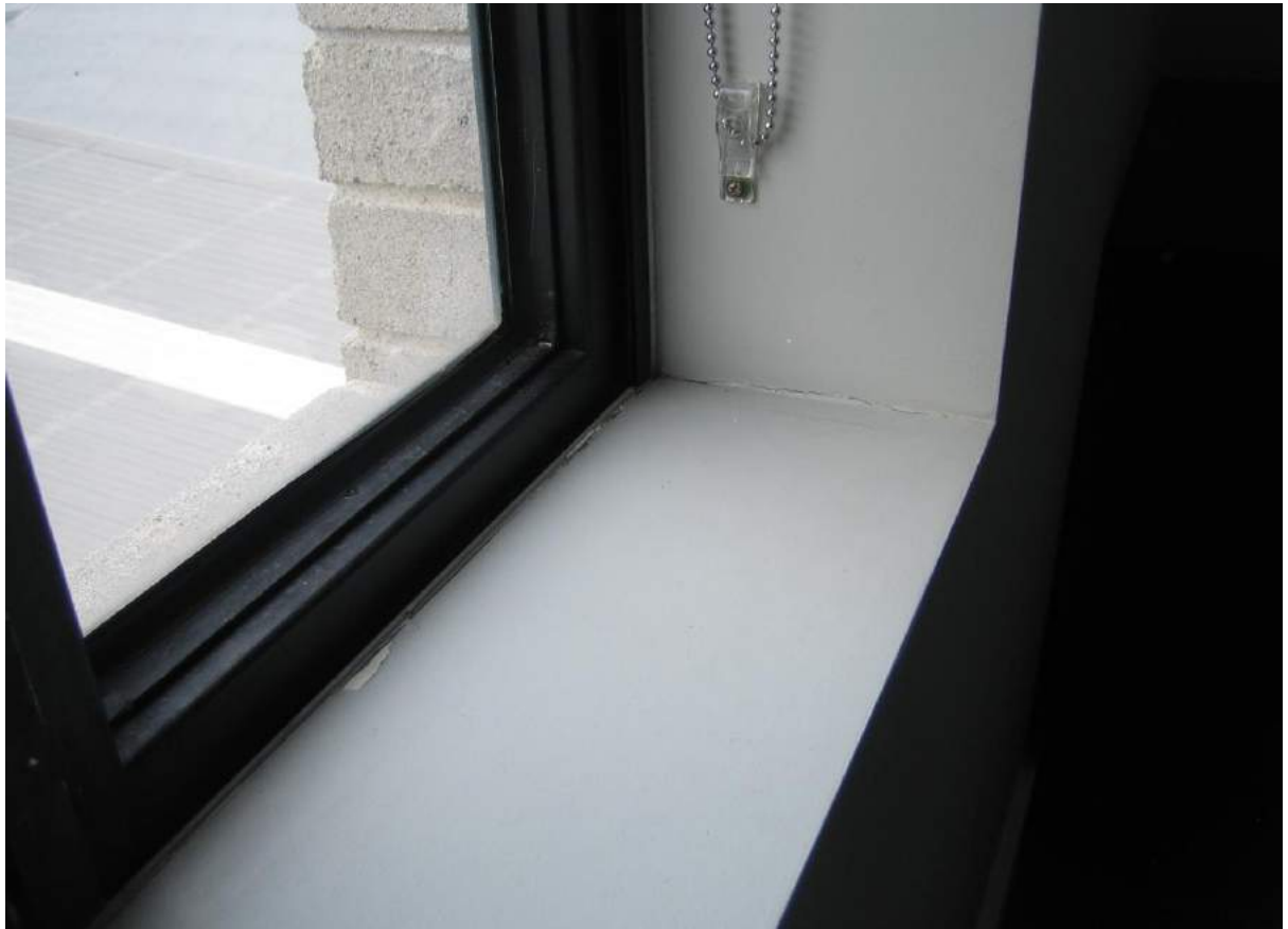
Photo No. 21: Water penetration and damage to the window sill in bedroom 2 in Unit 301.
