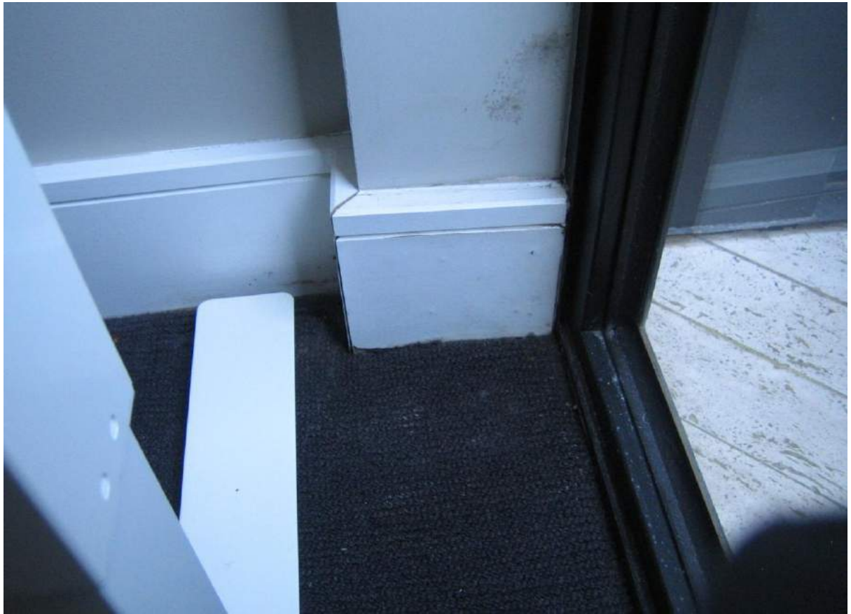
Photo No. 55: Water damage to skirting at eastern end of balcony door to Bed 3 to Unit 410.
