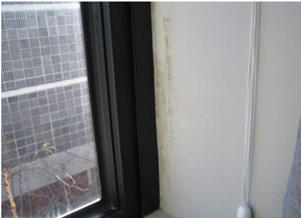
Photo No. 24: Water penetration in window in the N/E corner of bedroom 1 to Unit 305.
