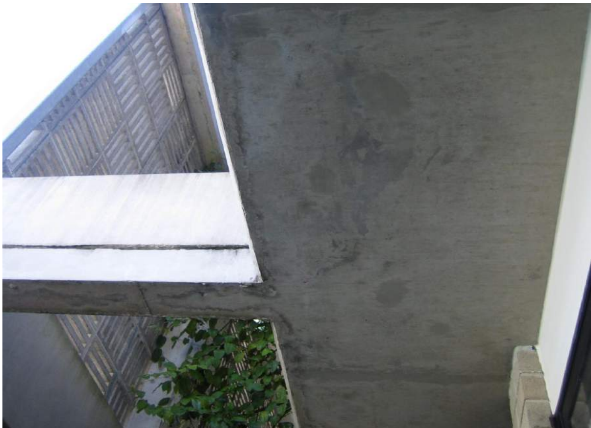
Photo No. 16: Soffit of balcony over bedroom 2 in Unit 212 has no drip-groove installed.
