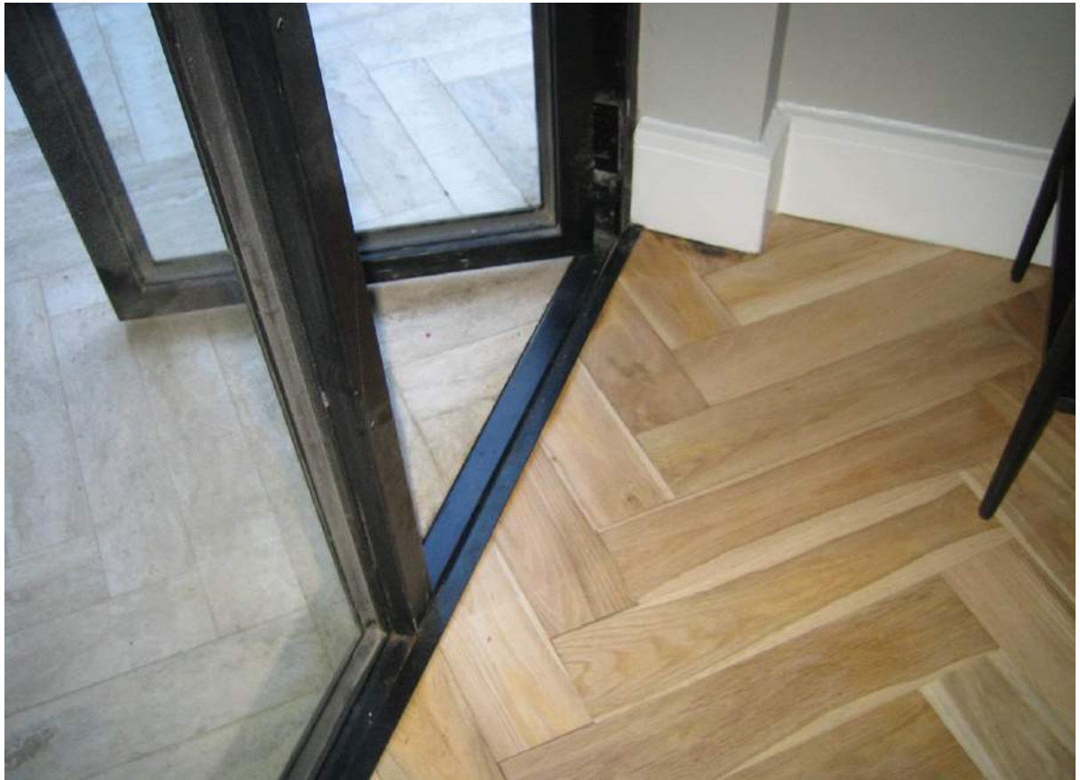
Photo No. 1: Water penetration and damage in N/W corner of bedroom 1 in Unit G01.
