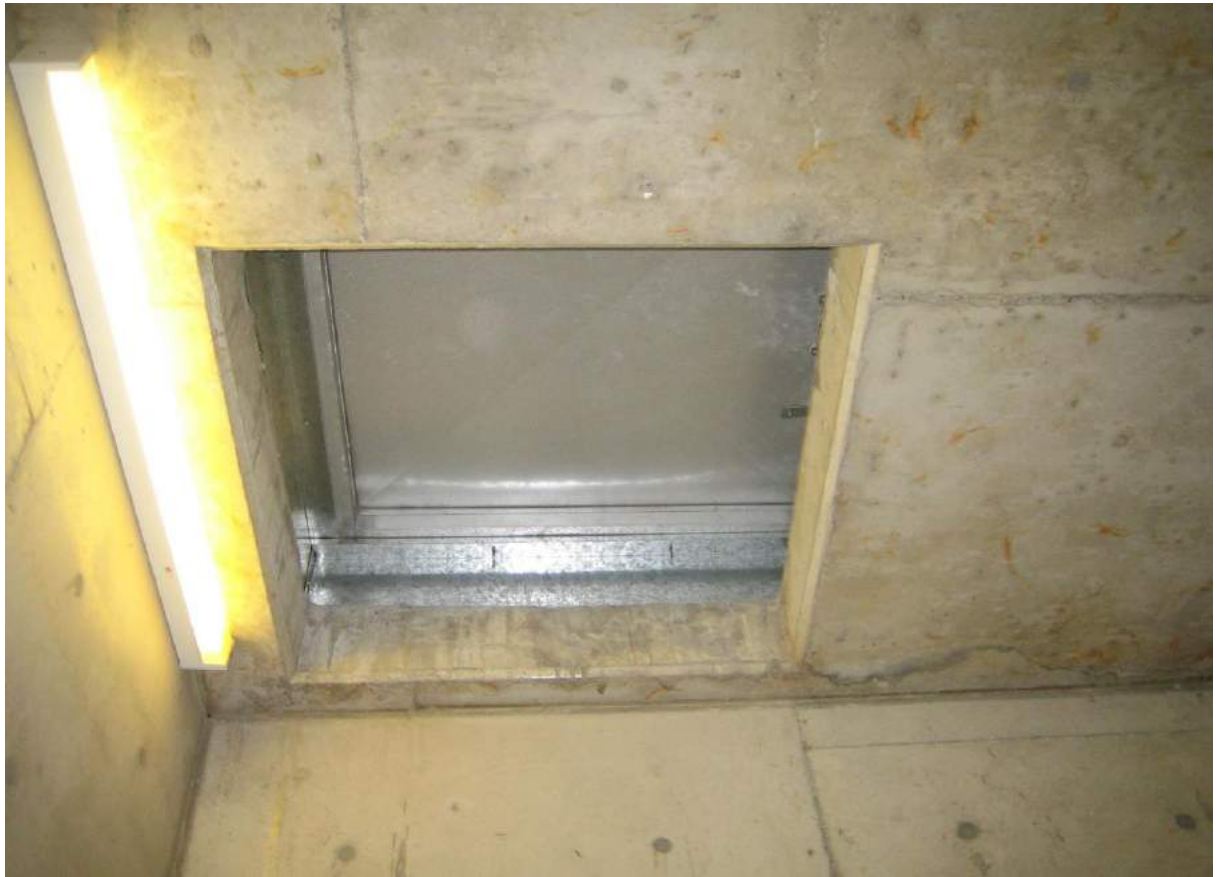
Photo No. 69: No fixed ladder for roof access on Level 4 of western fire stair in Building B.
