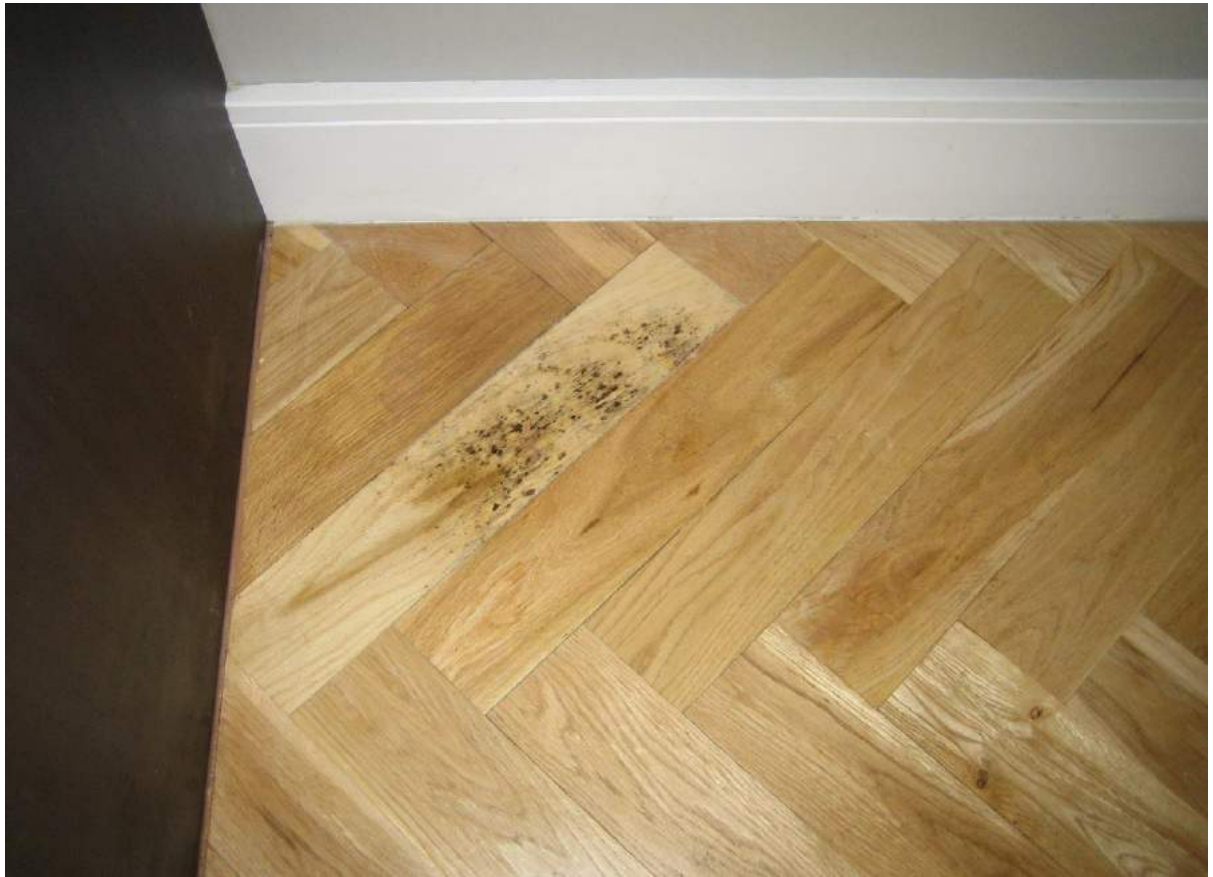
Photo No. 35: Mould stain in parquetry flooring in the kitchen within Unit 404.
