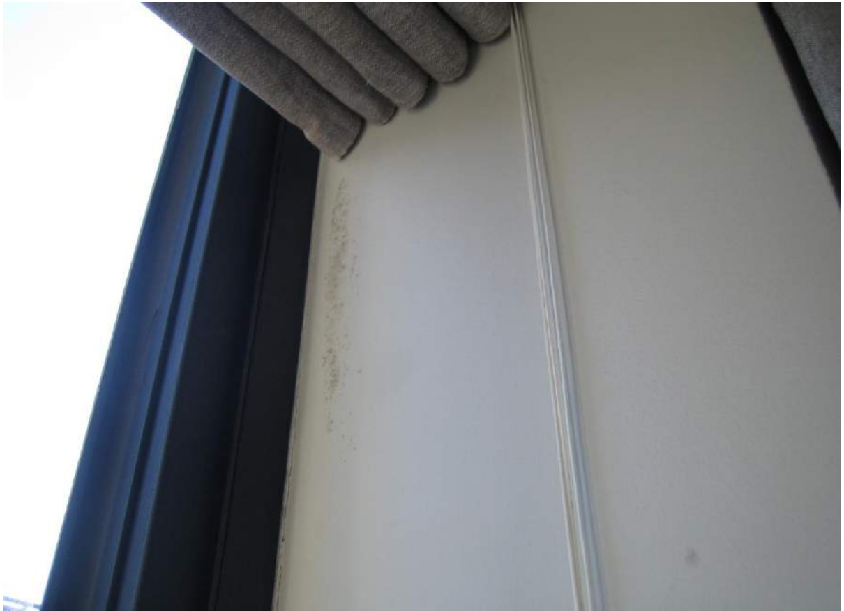
Photo No. 23: Water penetration in window in the N/E corner of bedroom 1 to Unit 305.
