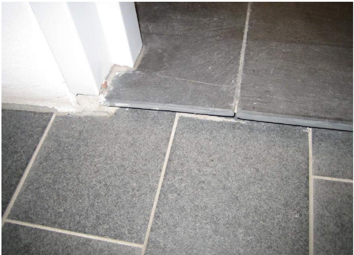
Photo No. 12: Front door tiled sill is cracked and not properly supported in Unit 106.
