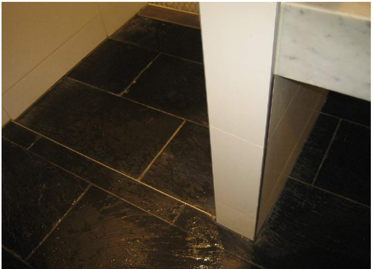
Photo No. 52: Water escapes the shower cubicle and ponds on tiled ensuite floor in Unit 409.
