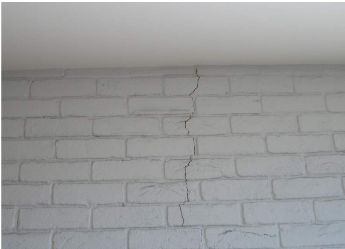
Photo No. 34: 1mm wide movement crack in the western balcony wall in Unit 312.
