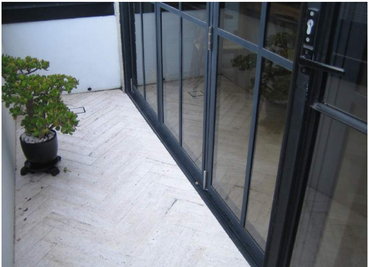
Photo No. 42: Water penetration and damage at living room balcony doors in Unit 406.
