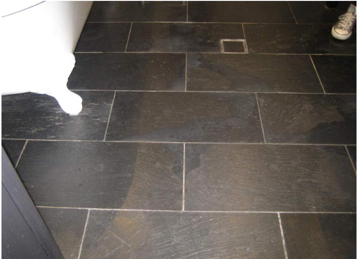
Photo No. 51: Water escapes the shower cubicle and ponds on tiled ensuite floor in Unit 409.
