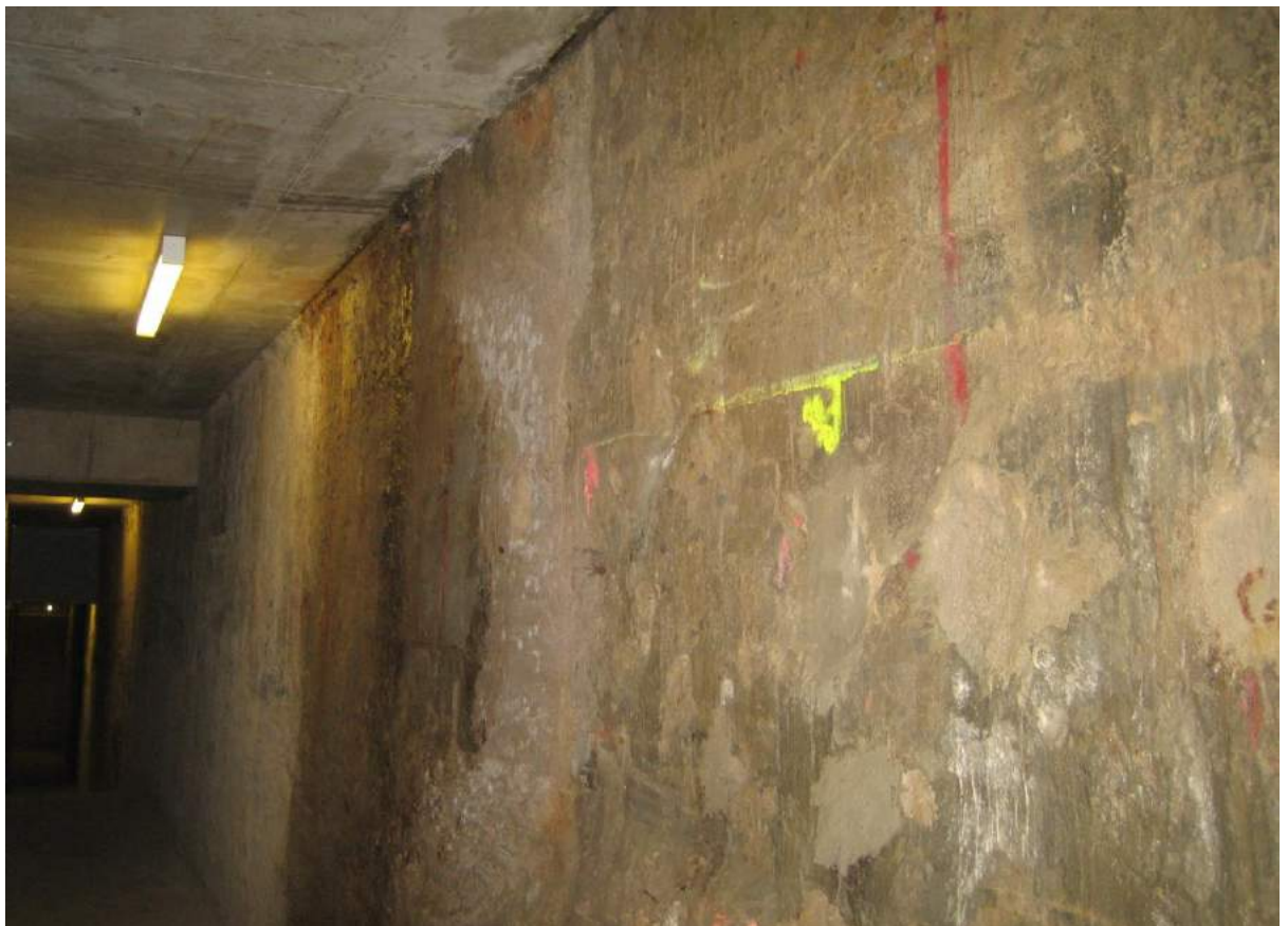
Photo No. 70: Water leaching in wall opposite Level B1 door in eastern fire stair in Building B.
