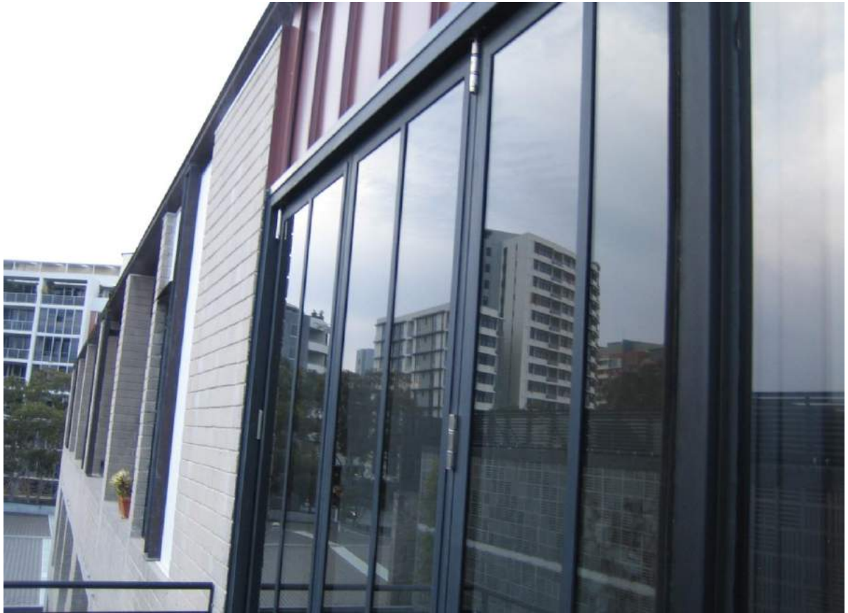
Photo No. 43: Exposed area over living room balcony door assembly in Unit 406.
