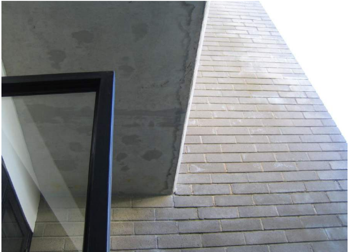
Photo No. 17: Soffit of balcony over bedroom 2 in Unit 212 has no drip-groove installed.
